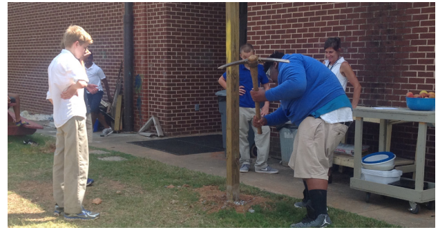
Ag Science students completing putting in a post for a shade structure at Clarke Middle School.
